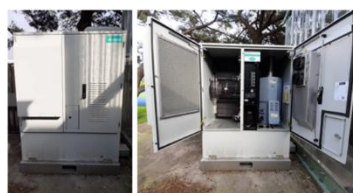
Hydrogen Fuel Cell
