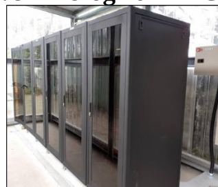
Storage Systems of MG2 and MG3
