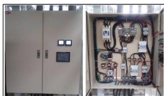
Switches of Interconnected System
